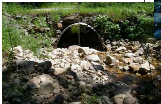
Undersized culvert at Langlois Creek Road Crossing, 2007.
