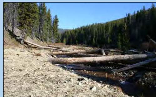
(10/29/08) Upper section of new channel - base flow only in stream for winter/spring 09.
