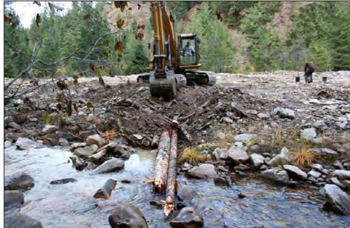
Installing logs and riparian plantings to enhance bank stability on the East Fork of Pine Creek, fall, 2008.
