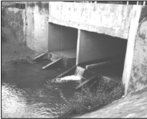
Figure 11. Photograph of Prefumo Creek, Fish Barrier PR-1-2B.
