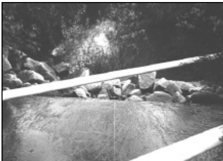
Figure 10. Photograph of Prefumo Creek, Fish Barrier PR-1-1B.
