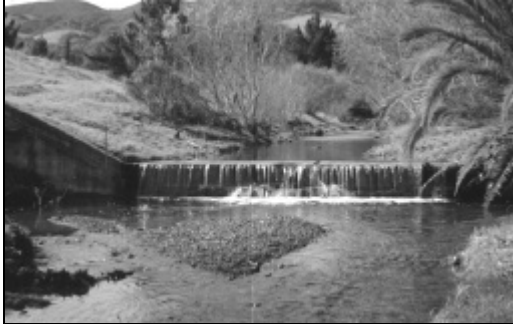
Figure 13. Photograph of Prefumo Creek, Fish Barrier PR-2-1B
