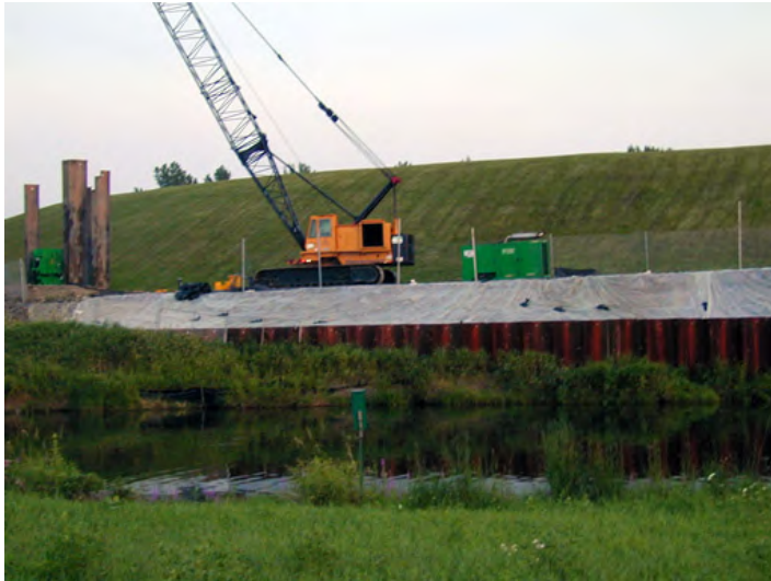
Turtle Cove prior to cleanup of PCB-contaminated sediments. The unlined 12-acre GM Landfill was capped with clay and seeded with grass.
